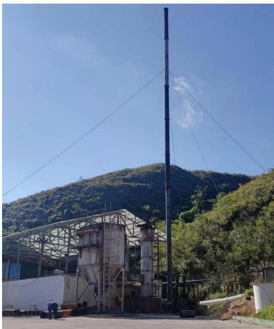
布袋除尘+碱洗脱硫+30mDA002 排气筒
